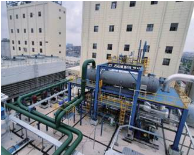
Figure 5 Overview of Exergy's ORC waste heat recovery installation at Sanfame's chemical plant
